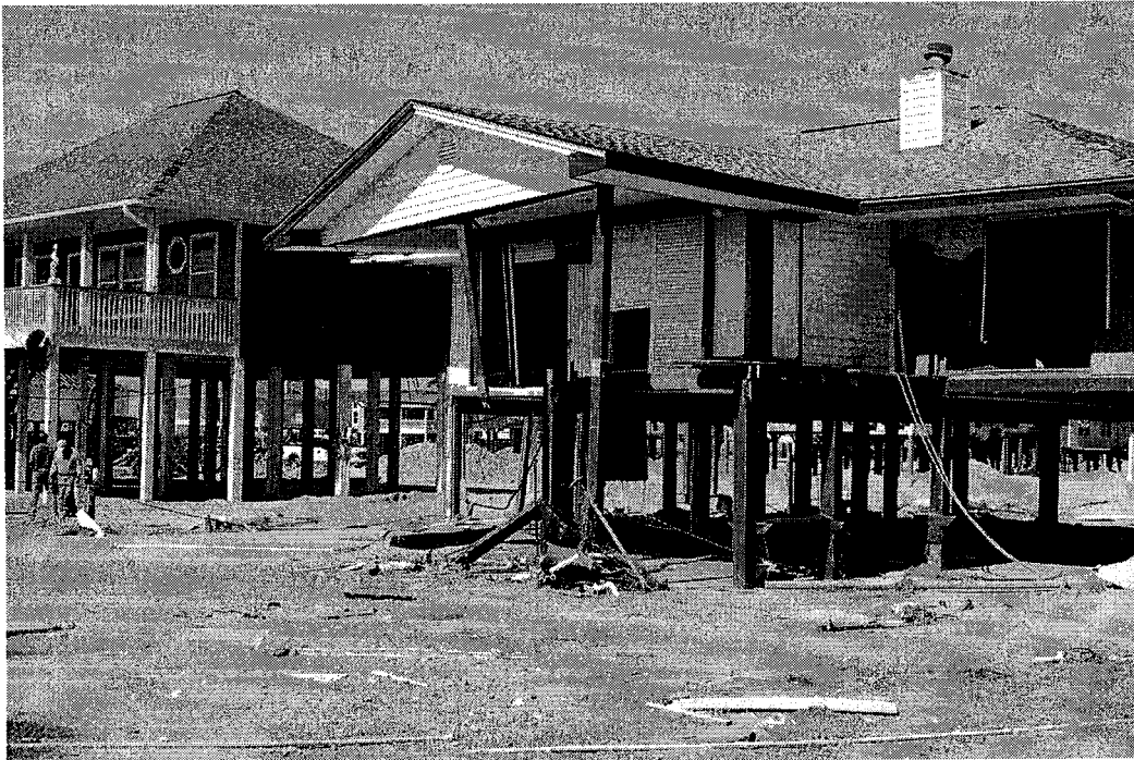
Figure 5. Bolivar Peninsula house on left sustained minor flood damage (to access stairs and below-BFE enclosures) during Ike, while the house on the right was severely damaged. The house on the left was constructed 5.5 ft above the BFE, the house on the right was estimated to be at the BFE (Oct. 18, 2008, photo C.P. Jones).
