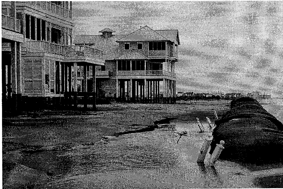
Figure 4. Erosion along the Galveston Island shoreline, west of the seawall (Oct. 17, 2008, photo C.P. Jones)
