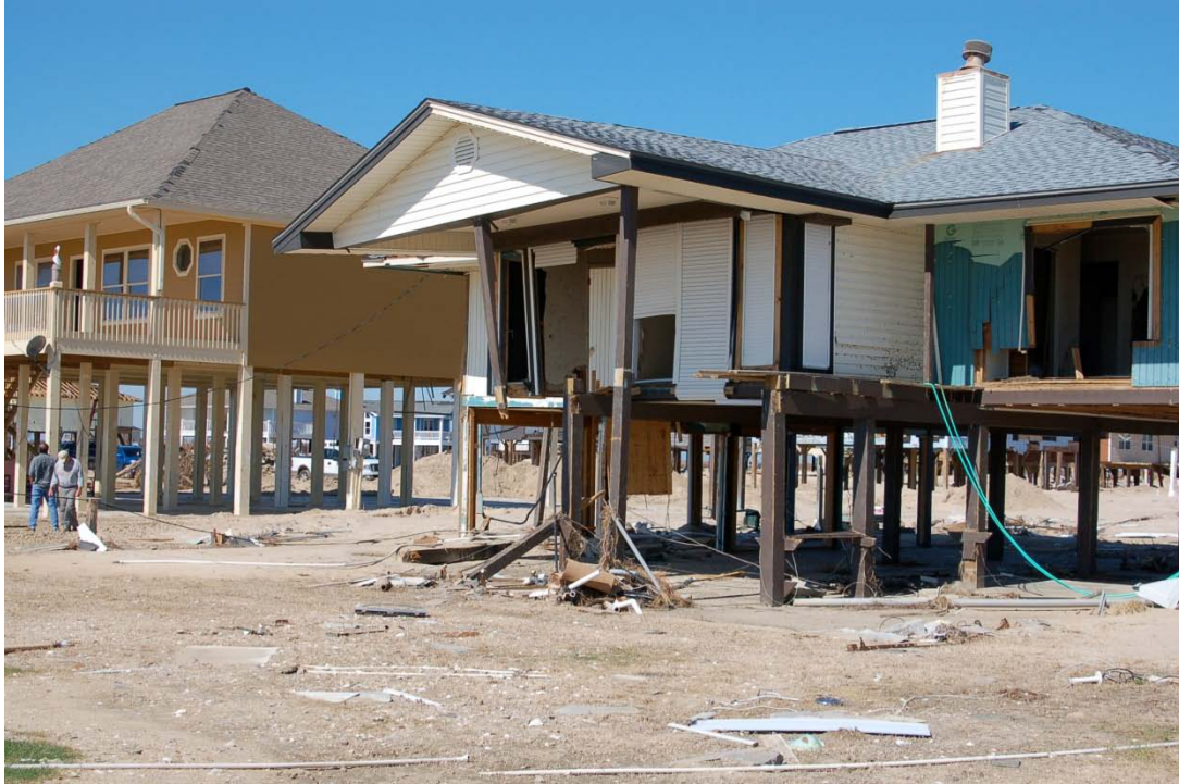
Figure 5. Bolivar Peninsula house on left sustained minor flood damage (to access stairs and below-BFE enclosures) during Ike, while the house on the right was severely damaged. The house on the left was constructed 5.5 ft above the BFE, the house on the right was estimated to be at the BFE (Oct. 18, 2008, photo C.P. Jones).
